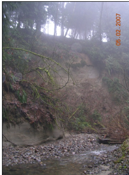
Photo 1: Large Slope Erosion with Houses near Slope Crest, an Example of Undercutting and Slab Regression.
