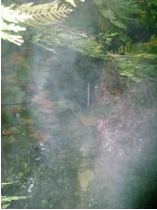
PHOTO 14 – Residential drainage pipe outletting onto slope
