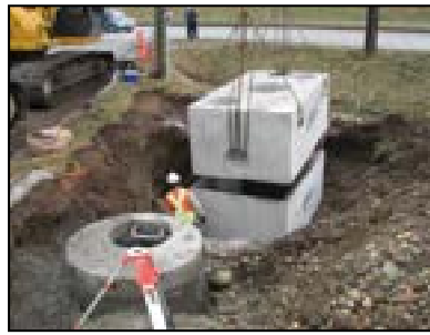
Oil Grit Separator
