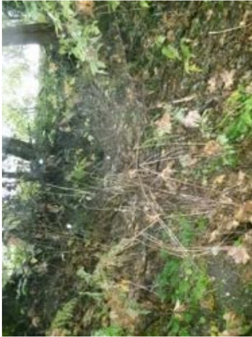
PHOTO 6 – Slope erosion above creek
