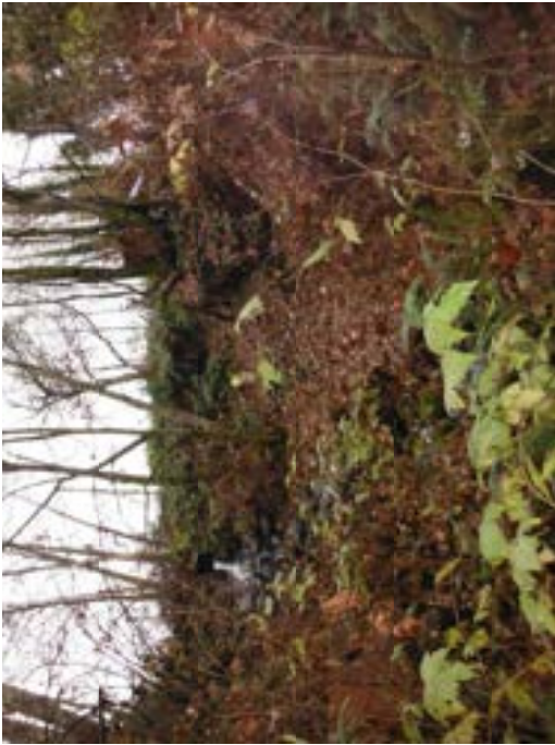
PHOTO 5 – Outfall east end of ravine, eroded left bank
