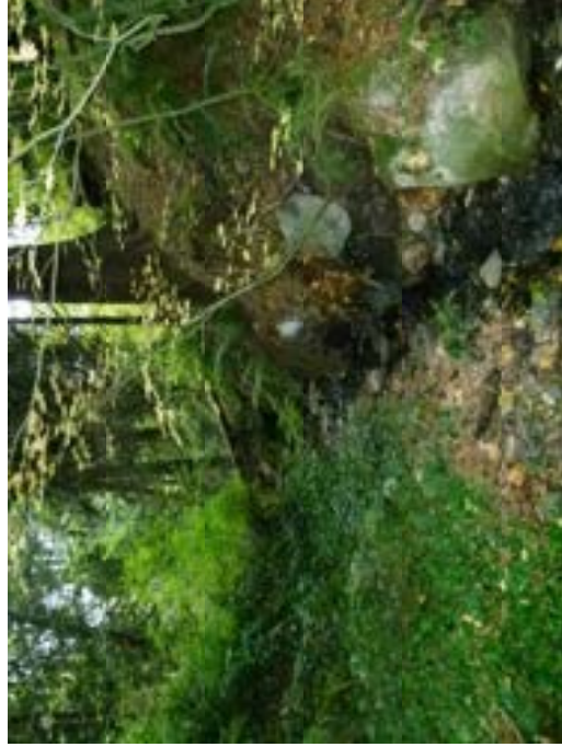
PHOTO 8 – Eroding north bank
