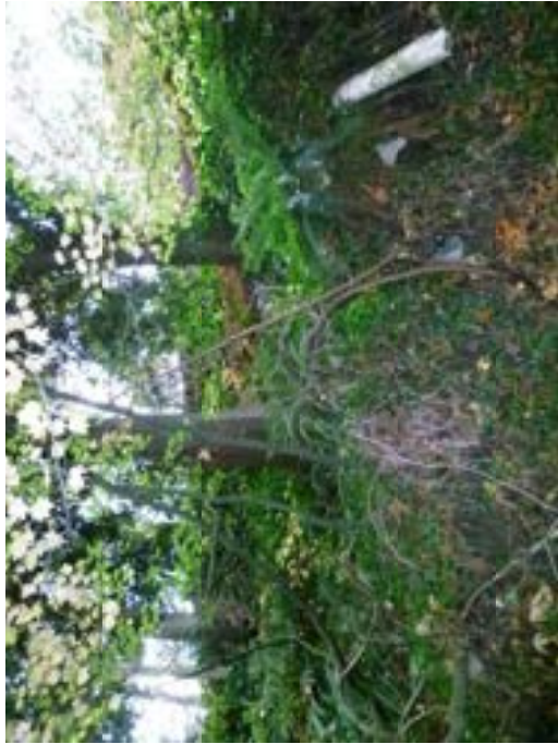
PHOTO 9 – Outfall pipe with sloughing fill
