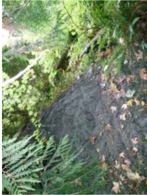
PHOTO 7 – Eroded bank exposing dense Silty Clay
