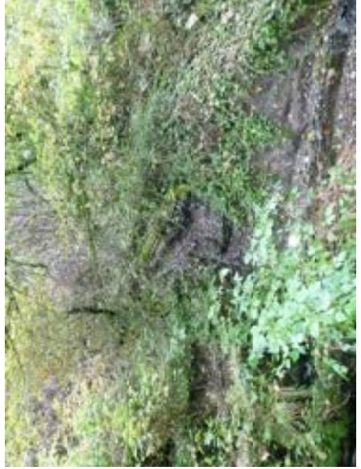
PHOTO 24 – Seepage at gully base south slope
