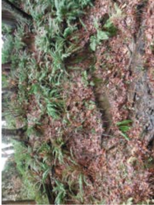
PHOTO 6 - Erosion of creek bank exposing Sand
