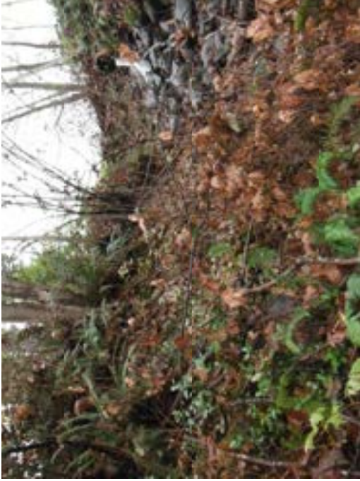
PHOTO 6 - Eroded right bank near outfall
