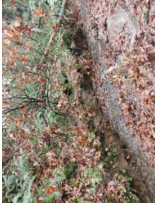
PHOTO 4 - Eroded banks exposing dense Silty Sand with some Gravel
