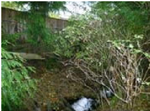
Undercutting of fence in McAdam Creek downstream of flow split chamber
