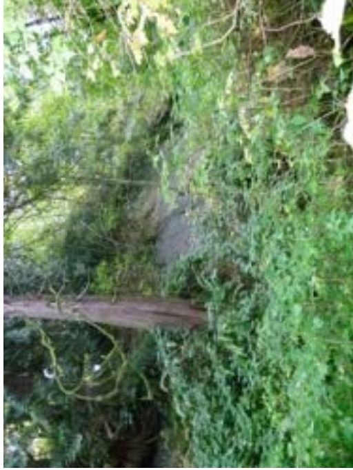
PHOTO 6 - Failing north bank
