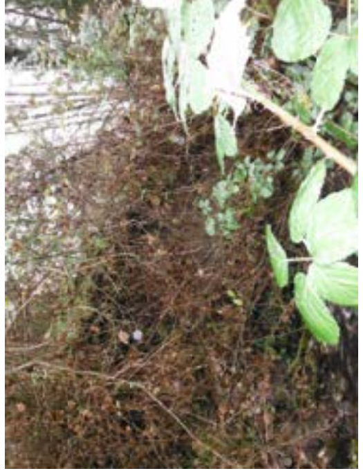
PHOTO 4 – Eroded bank on outside of creek bend
