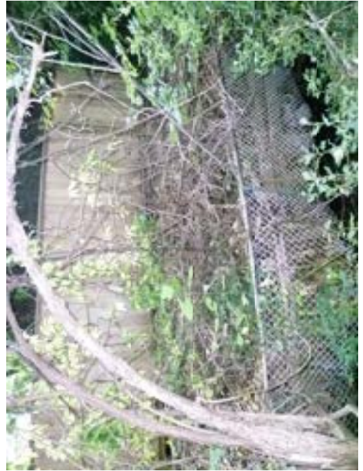
PHOTO 3 – Fence in water, potential blockage
