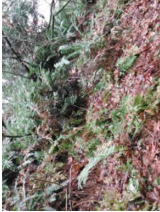
PHOTO 12 – Minor scarps near slope toe
