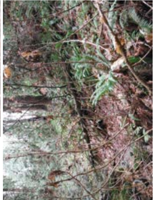
PHOTO 7 – Slide scarp at slope toe north bank
