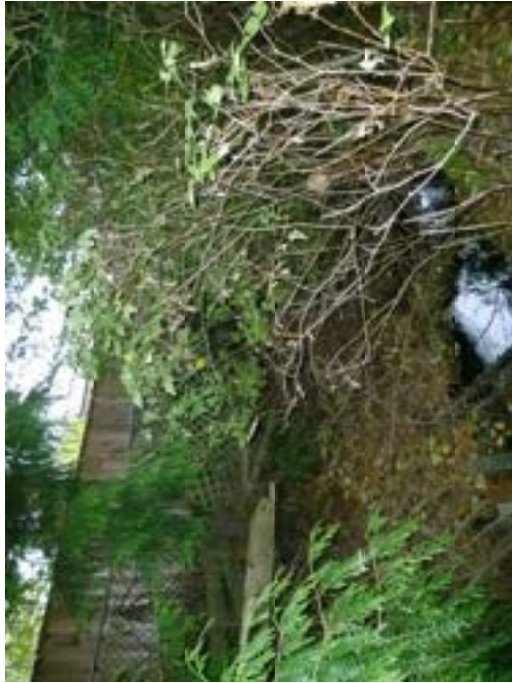
PHOTO 1 – Undermined fence south bank
