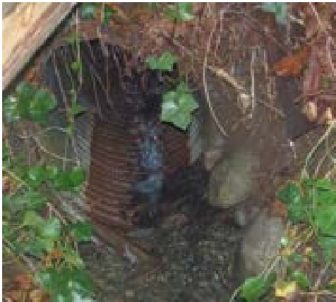
Eroded culvert on Collings Creek
