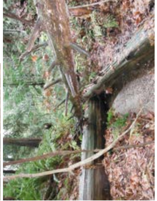
PHOTO 8 – Fallen trees creating blockage
