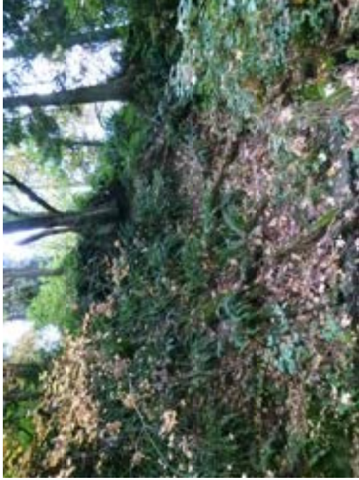
PHOTO 22 – Steep bank undermining crest
