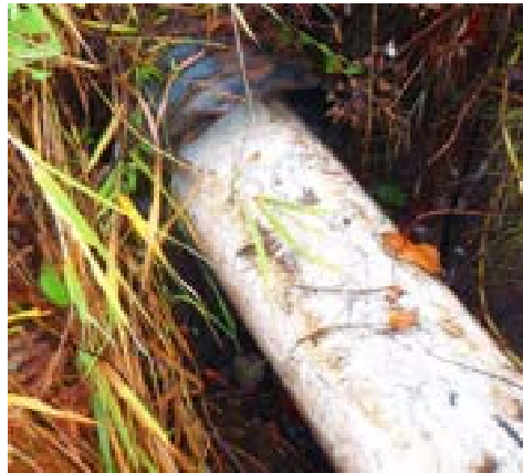
Projecting Outfall between Norum and Collings Creek causing erosion of bank
