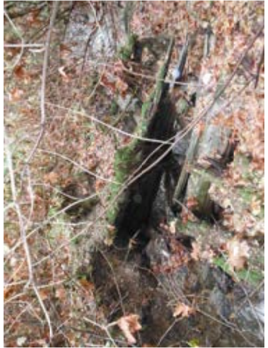
PHOTO 15 – Tree down in creek, potential blockage
