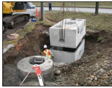
Oil Grit Separator
