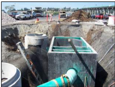
Oil Grit Separator
