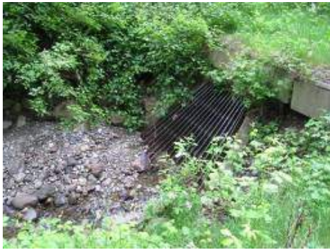
Sediment/debris in Shaw Creek at upstream end of Highway 10 culvert
