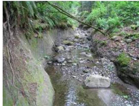
Bank Erosion in Shaw Creek downstream of Highway 10 culvert
