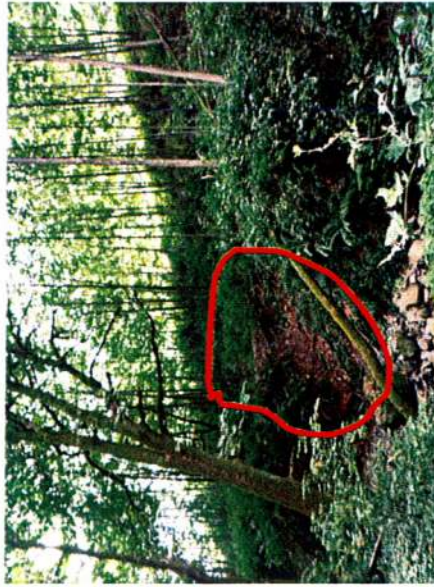
PHOTO 15 – Abandoned Dirt Road – Note Slough Resulting From Undermining
