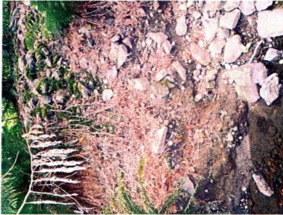
PHOTO 21 – Eroded Rip Rap Bank From Abandoned Road Crossing
