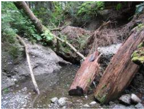
Debris Jams in Shaw Creek between 120 Street and Highway 10
