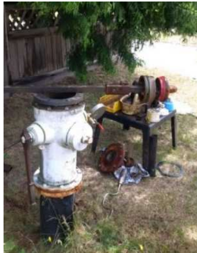
Figure 12: Fire Hydrant Undergoing Regular Annual Maintenance
