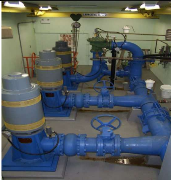
Figure 9: Pump Station on 4 Avenue at Pebble Hill Reservoir
