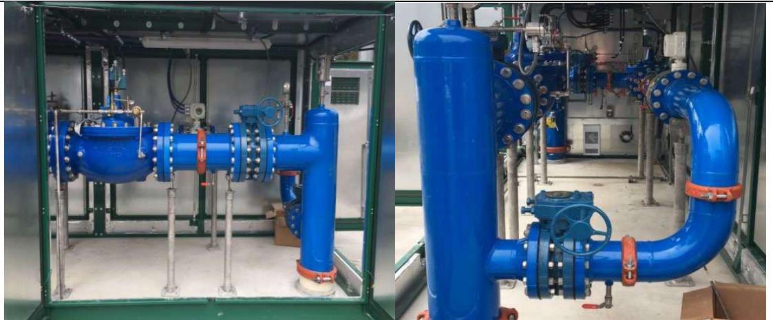
Figure 11: Norum Road PRV Station
