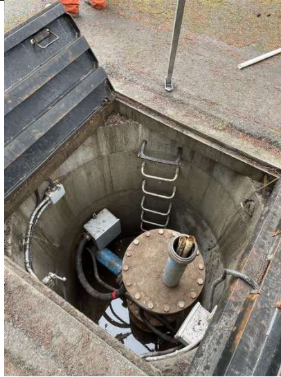
Figure 14: Well #5, Watershed Park Wells
